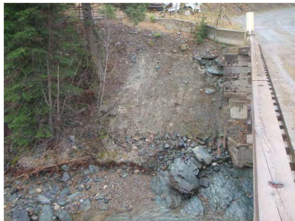
Figure 1-16: Downstream woods end embankment, note erosion at toe of embankment.
