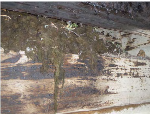
Figure 1-15: Debris accumulation on woods end cap beam.
