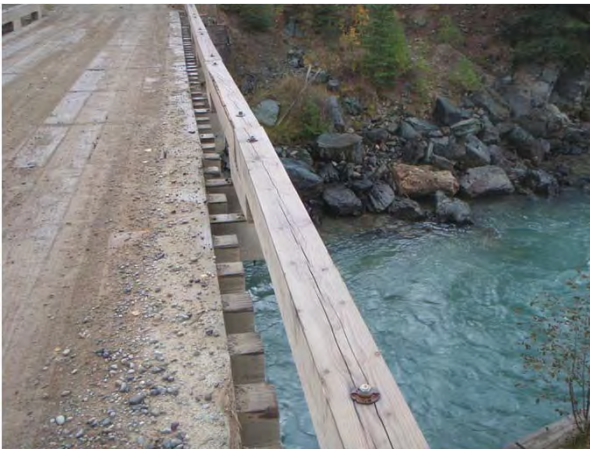
Figure 1-7: Typical curb rail condition.
